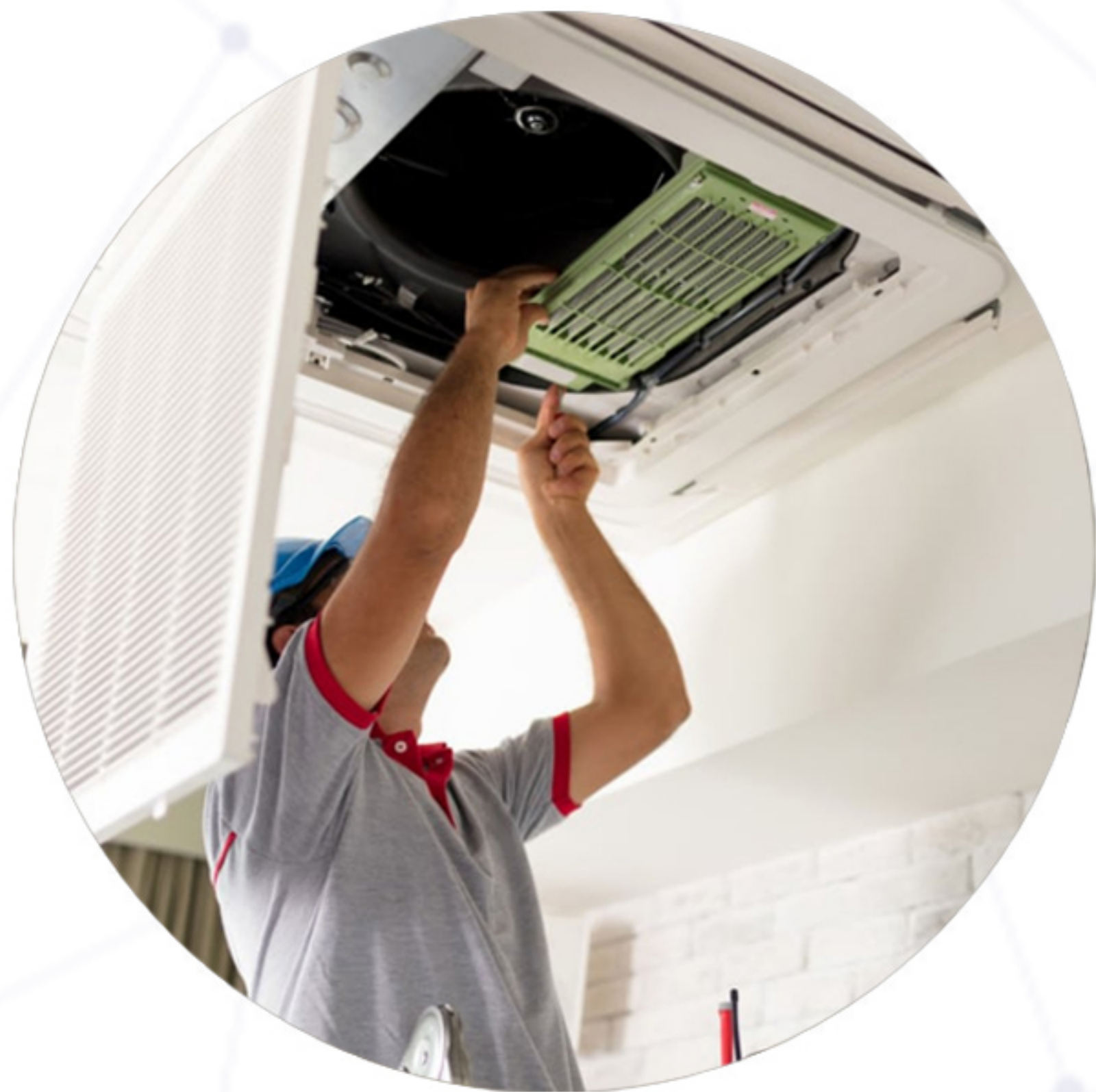
Air-condition And plant maintenance.
